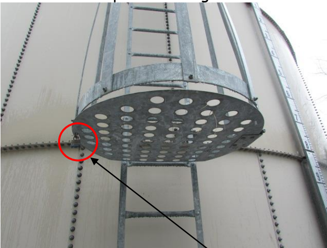
Tank ladder is caged and kept locked
