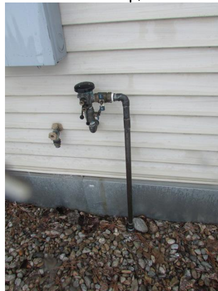
Pressure vacuum breaker on treatment plant building for surrounding lawn.
