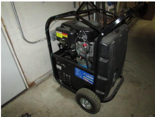
Generator is available in treatment plant building
