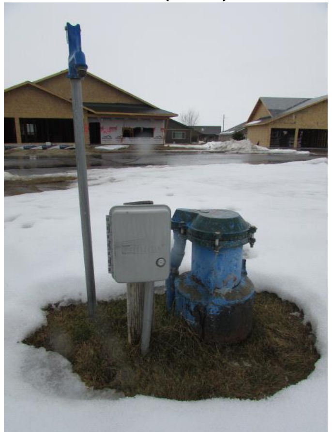
Well 2 with frost free hydrant
