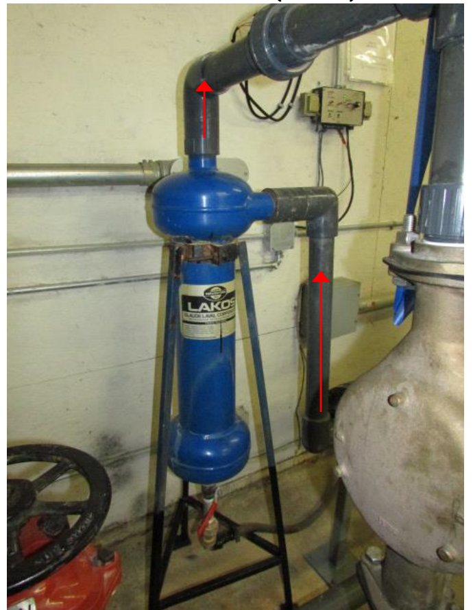
TP for Wells (TP001) step 1: A Lakos sand separator unit
