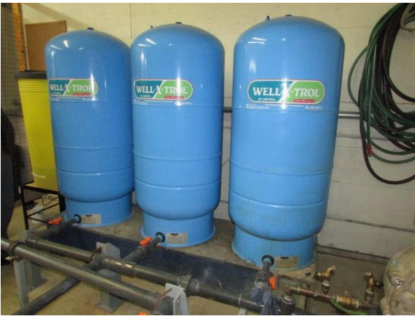
Pressure Control component - Three pressure tanks
