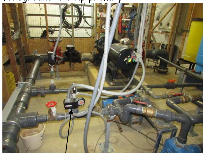
Pressure transducer for distribution is just after PC001 pumps
