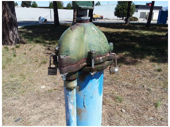
Photo of Well 1 received 5/3 showing new bolts in place (one had been missing)
