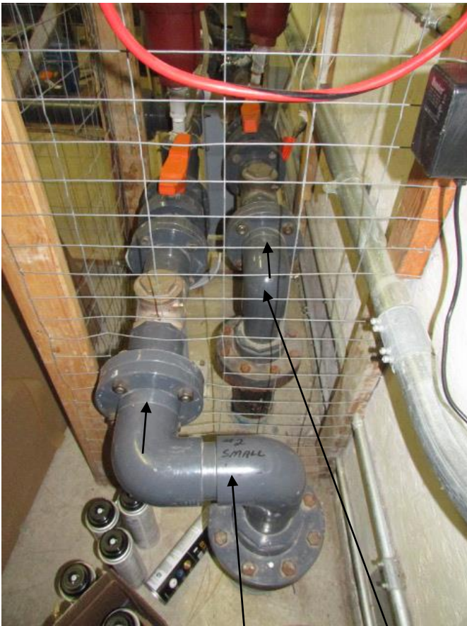
Incoming lines from Well 2 and Well 1
