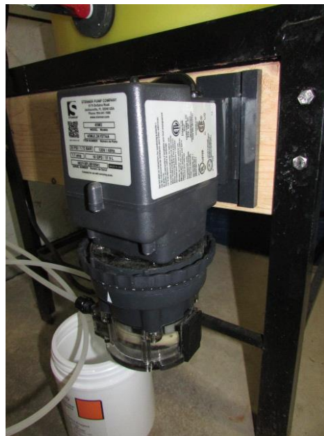
Chemical pump - Stenner peristaltic pump
