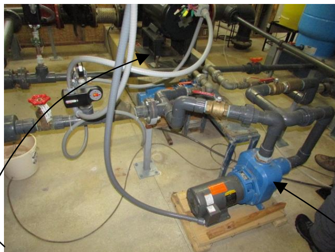
Pressure Control (PC001) - Two jet pumps, rear pump is 2 hp back up, and pump in foreground is 5 hp primary
