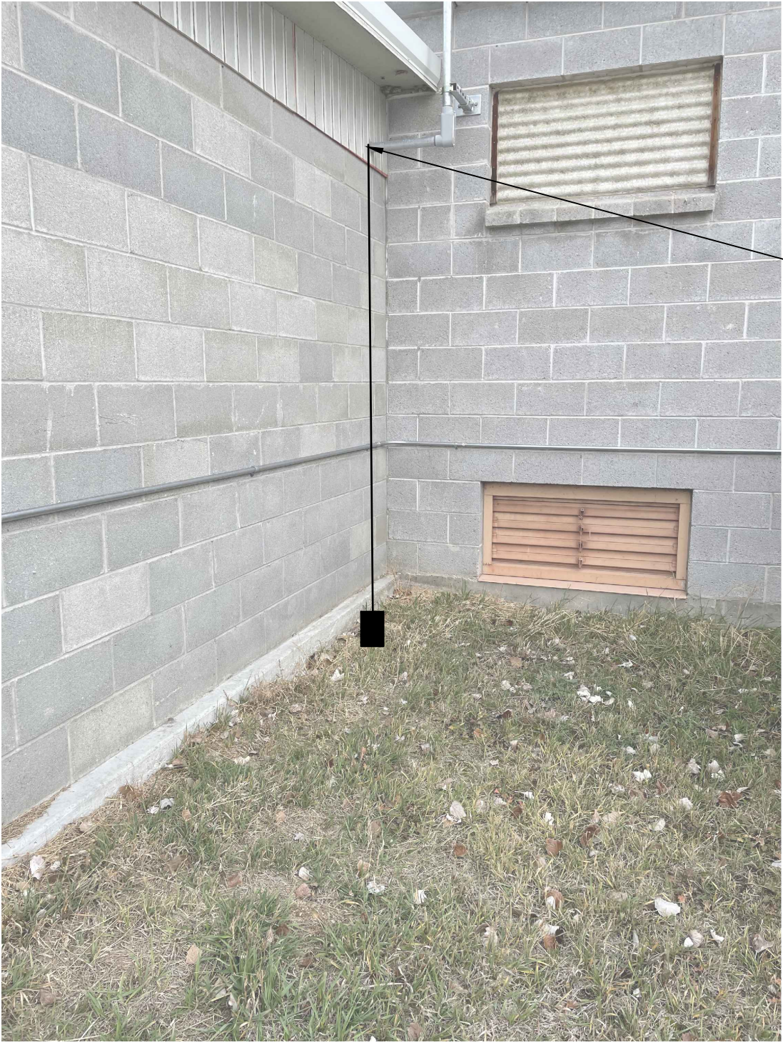
2 EXISTING ANTENNA CONDUIT VIEW 200E-02 NOT TO SCALE
