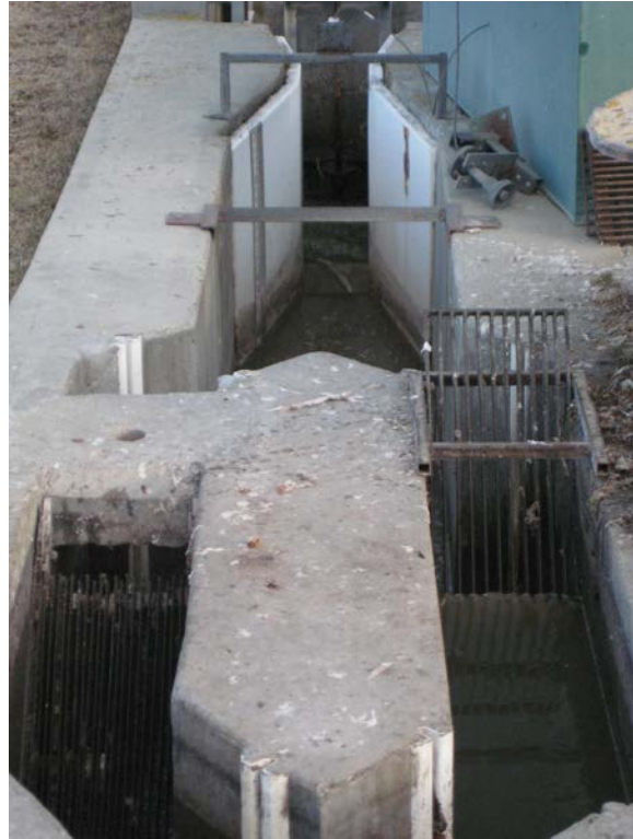
Figure II-1 Photograph of influent screen and Parshall flume showing the modifications to the screen on the left.
