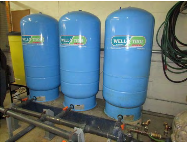
Pressure Control component - Three pressure tanks
