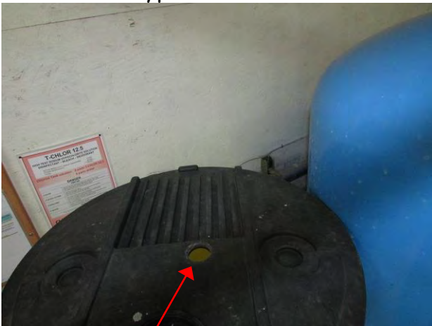
Batch tank was open - this should be closed
