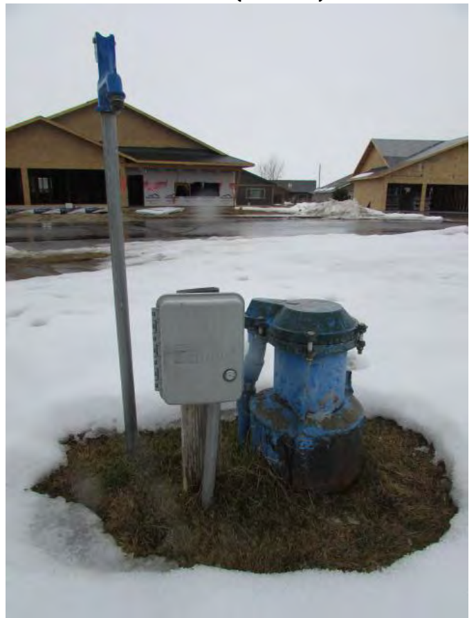
Well 2 with frost free hydrant
