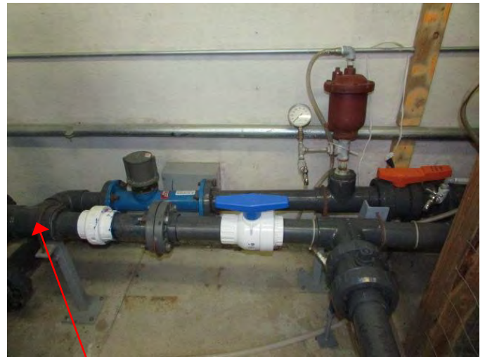
Common Header Well 1 2 (CH001)
