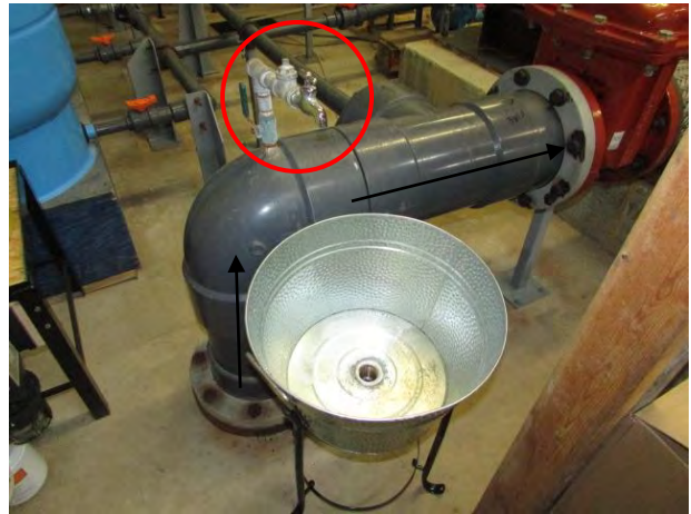
Line from ST001 to PC001 with sample tap in between
