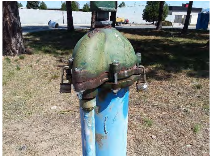
Photo of Well 1 received 5/3 showing new bolts in place (one had been missing)
