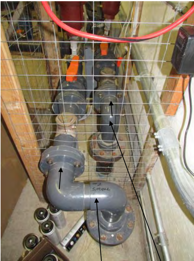
Incoming lines from Well 2 and Well 1
