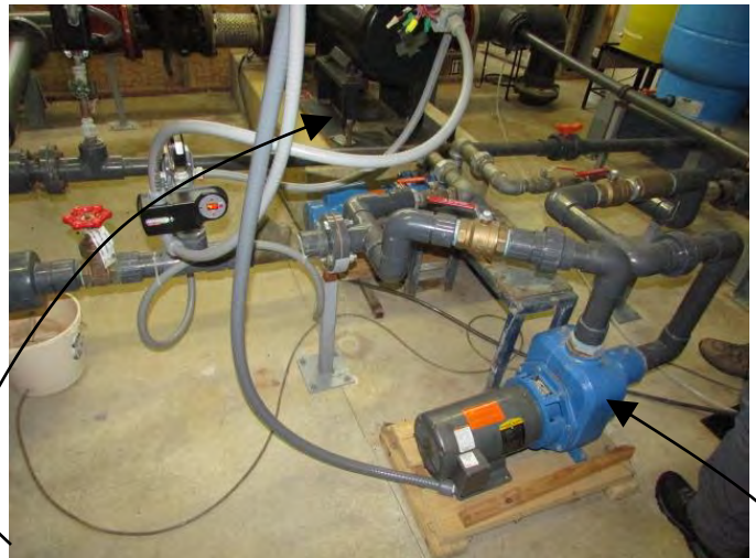
Pressure Control (PC001) - Two jet pumps, rear pump is 2 hp back up, and pump in foreground is 5 hp primary
