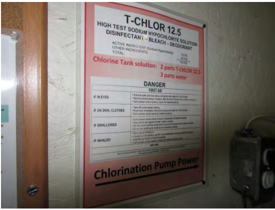
T-Chlor information on the wall
