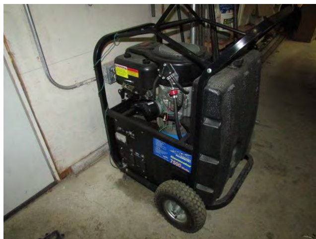
Generator is available in treatment plant building
