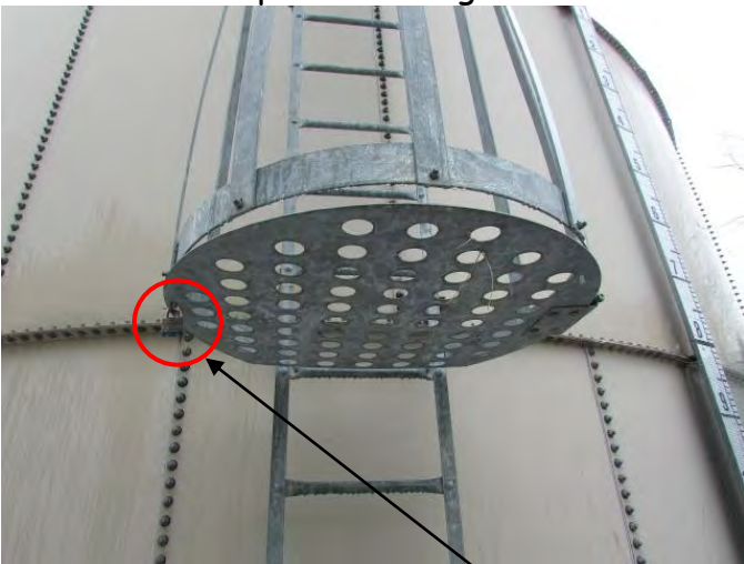
Tank ladder is caged and kept locked
