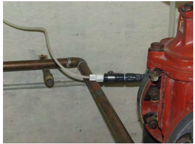
Injection quill on line as it enters ST001
