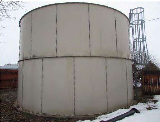
Storage Tank (ST001) is located just behind the Treatment plant building
